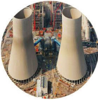
Armenia Power Plant
